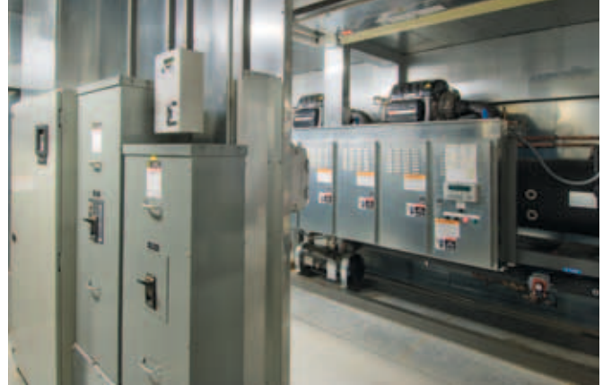
Chillers and Chiller Plants
