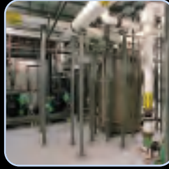
Boilers and water heaters are easily integrated
