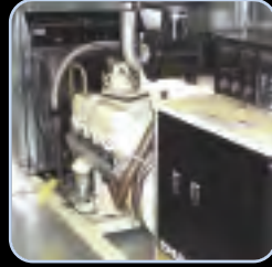
An ideal location for standby generators
