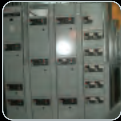
Electrical control centers and DDC options
