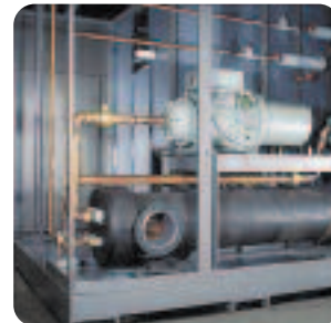
DX cooling with water-cooled condenser
